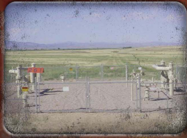
▲ VALVE YARD – NO GAS FLOWING
